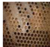
A badly scaled/fouled heat exchanger
